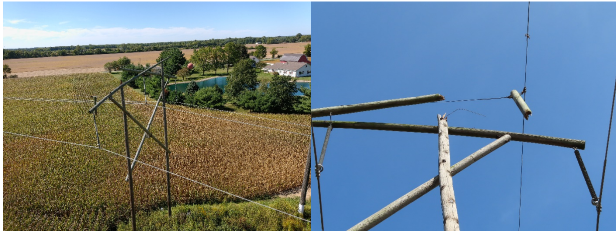
Figure 1: Broken Utility Pole
