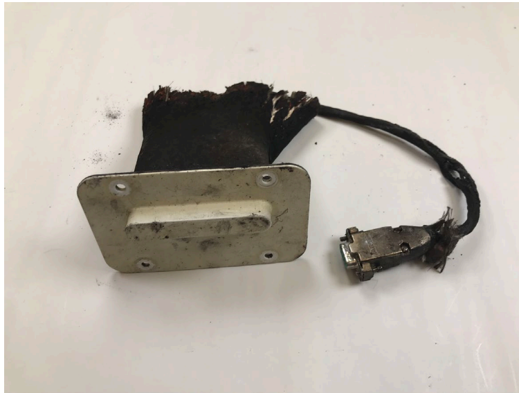
Figure 1. Photo of heat and smoke damaged RDM unit.
