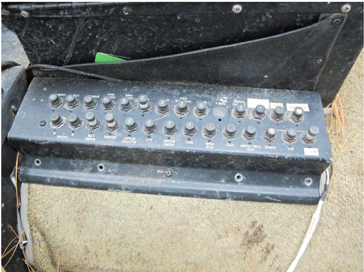
Circuit breaker panel.
