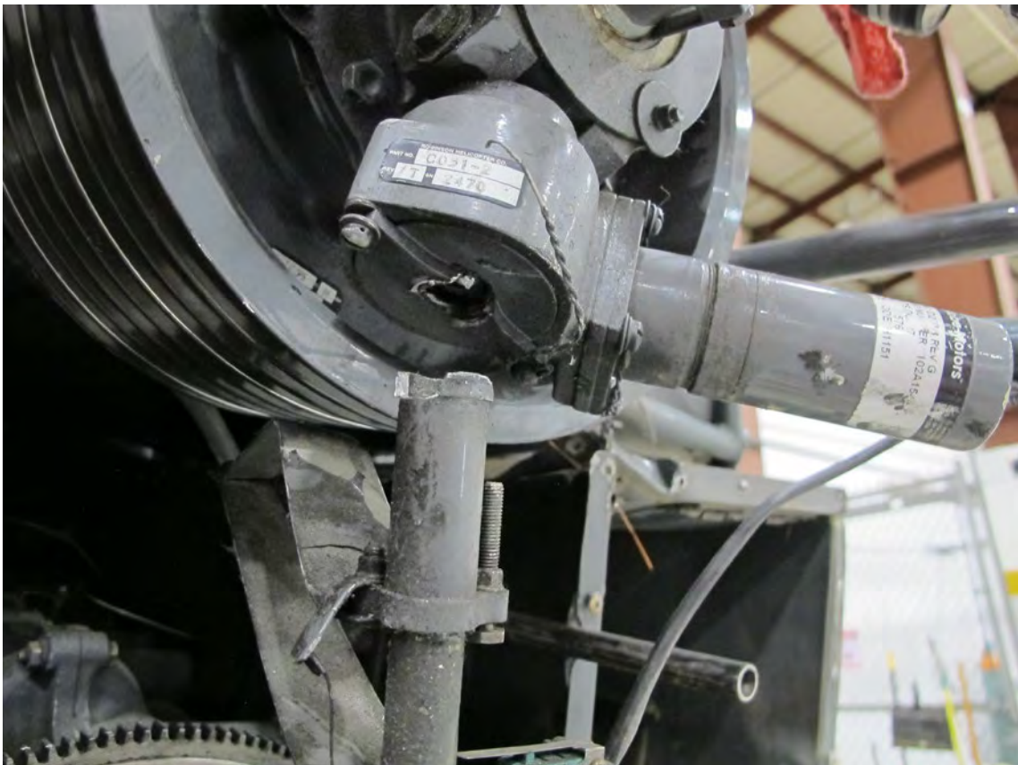
Disconnect in belt tension actuator.
