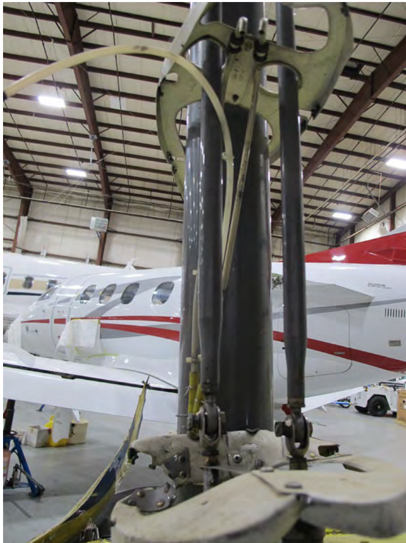
Fuel system vent tubes.
