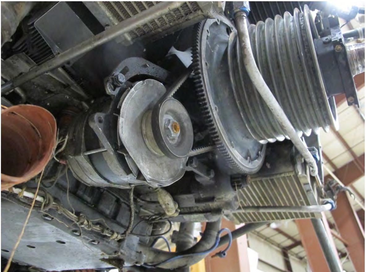
Damage to circumference of alternator cooling fan.
