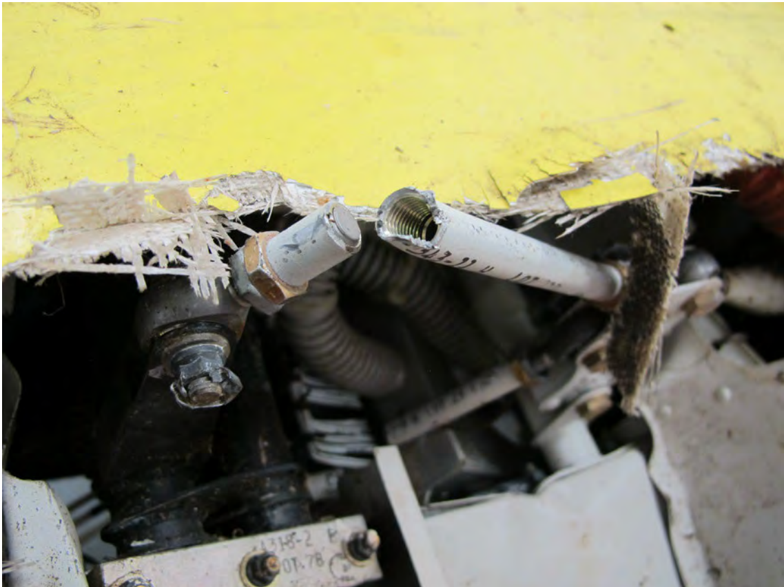
Disconnect TB in C343-11 push pull tube.
