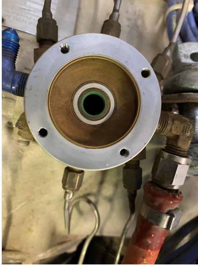
Figure 8, Fuel Distribution Manifold Screen
