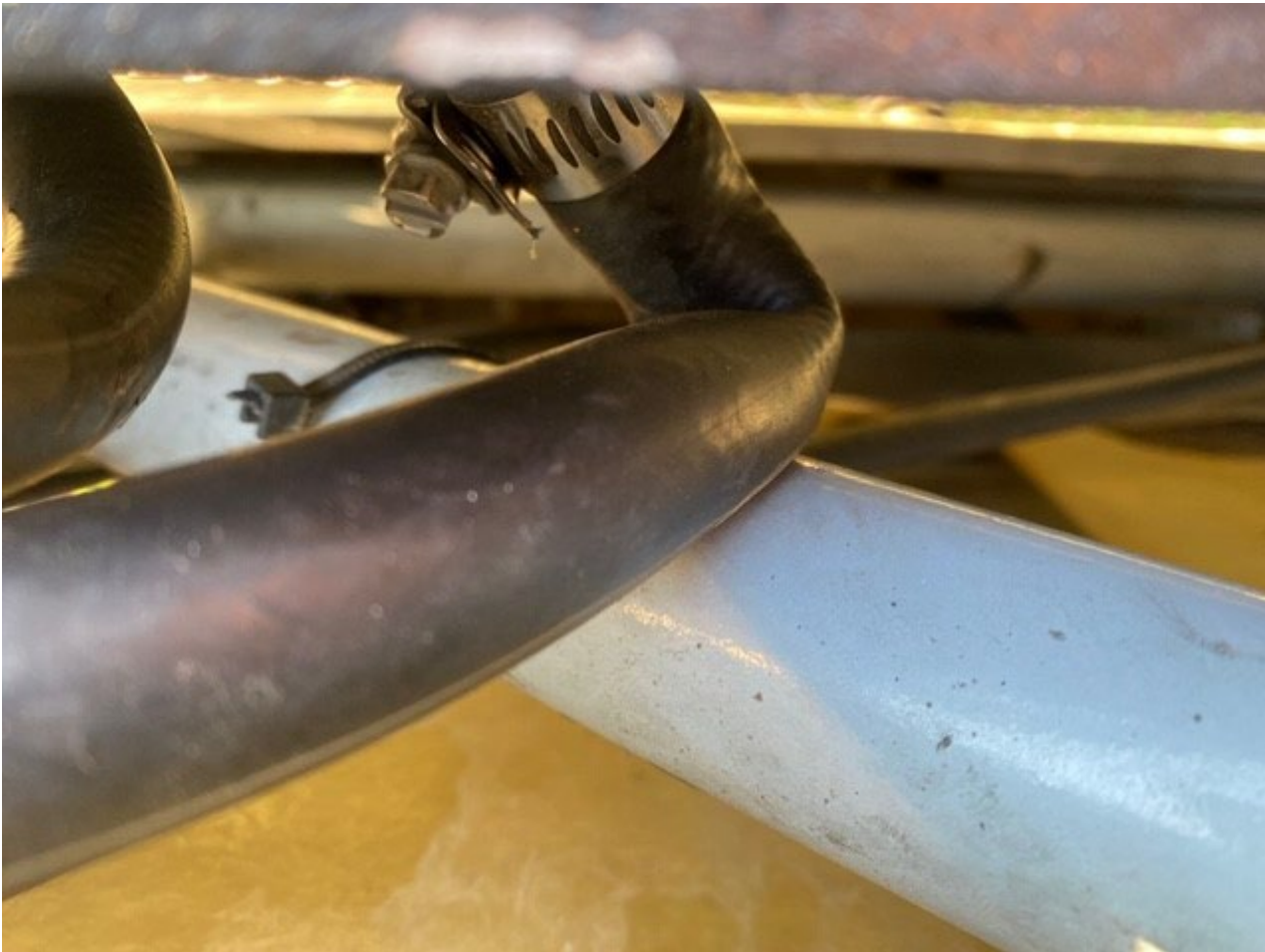
Kinked Fuel Vent Line
