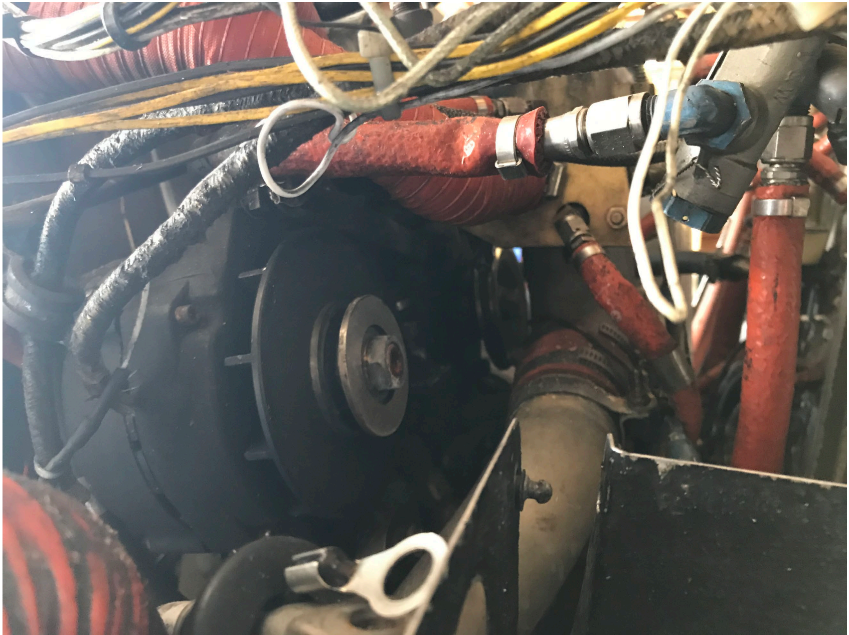
Photo 6 – View of Alternator – Missing Drive Belt
