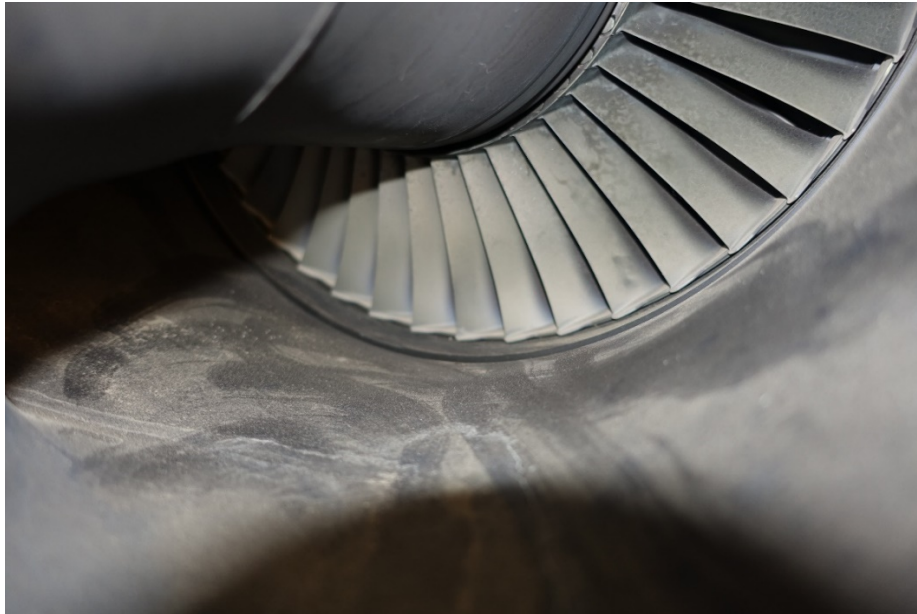
Photo 22- Trailing Edge, 2nd Stage Power Turbine Blades
