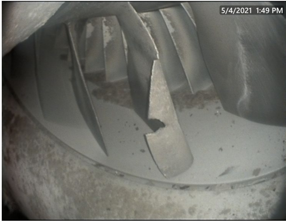
Photo 20- 1st Stage Compressor Blade Damage
