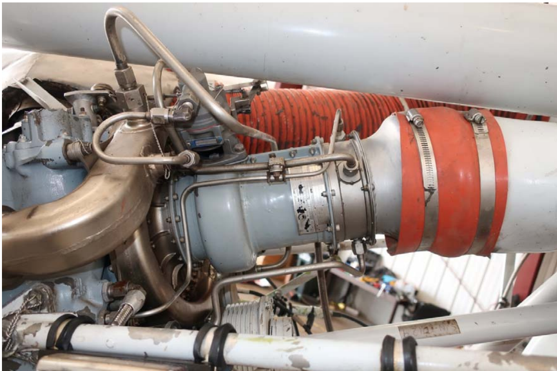
Figure 3. Compressor in-situ prior to field examination
