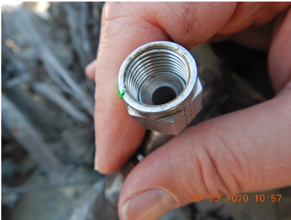
Photo 3 – Fuel pump inlet – shoulder of b-nut
