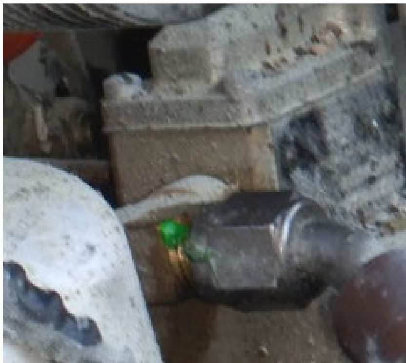
Photo 2 – Close up view of fuel inlet b-nut fitting
