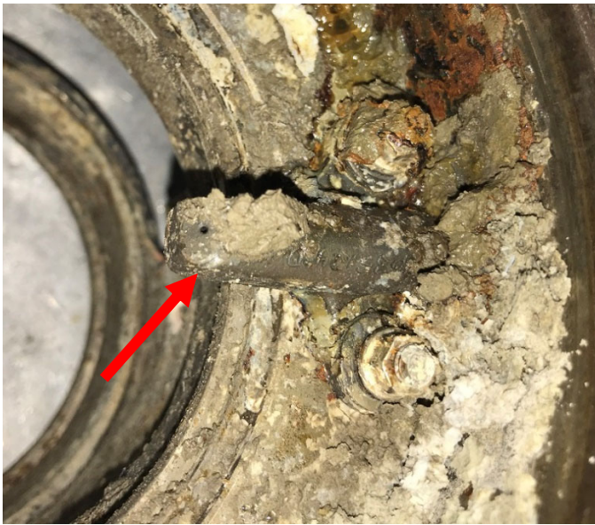
Figure 11. The oil nozzle (red arrow) located on the Nos. 3 and 4 bearing support housing.
