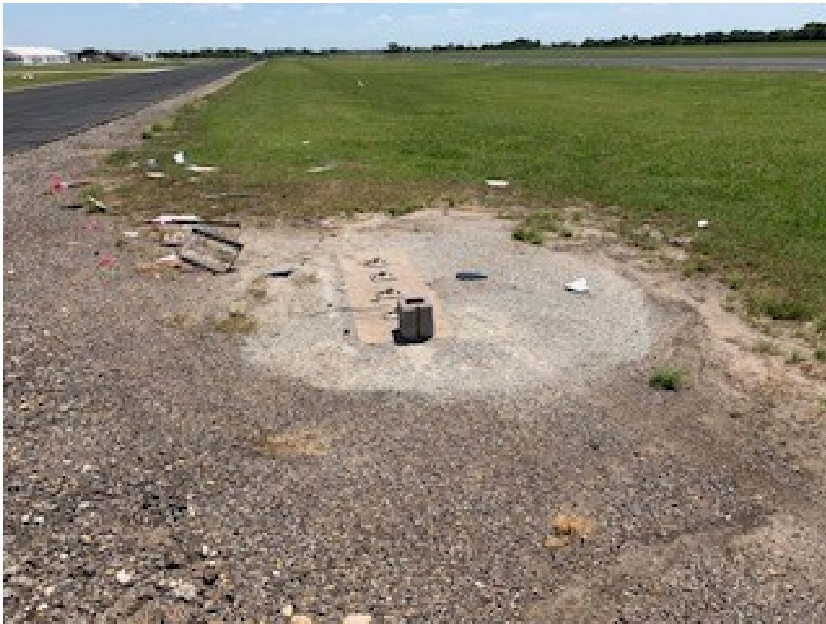
Photo 2 – Damaged Airport Sign
