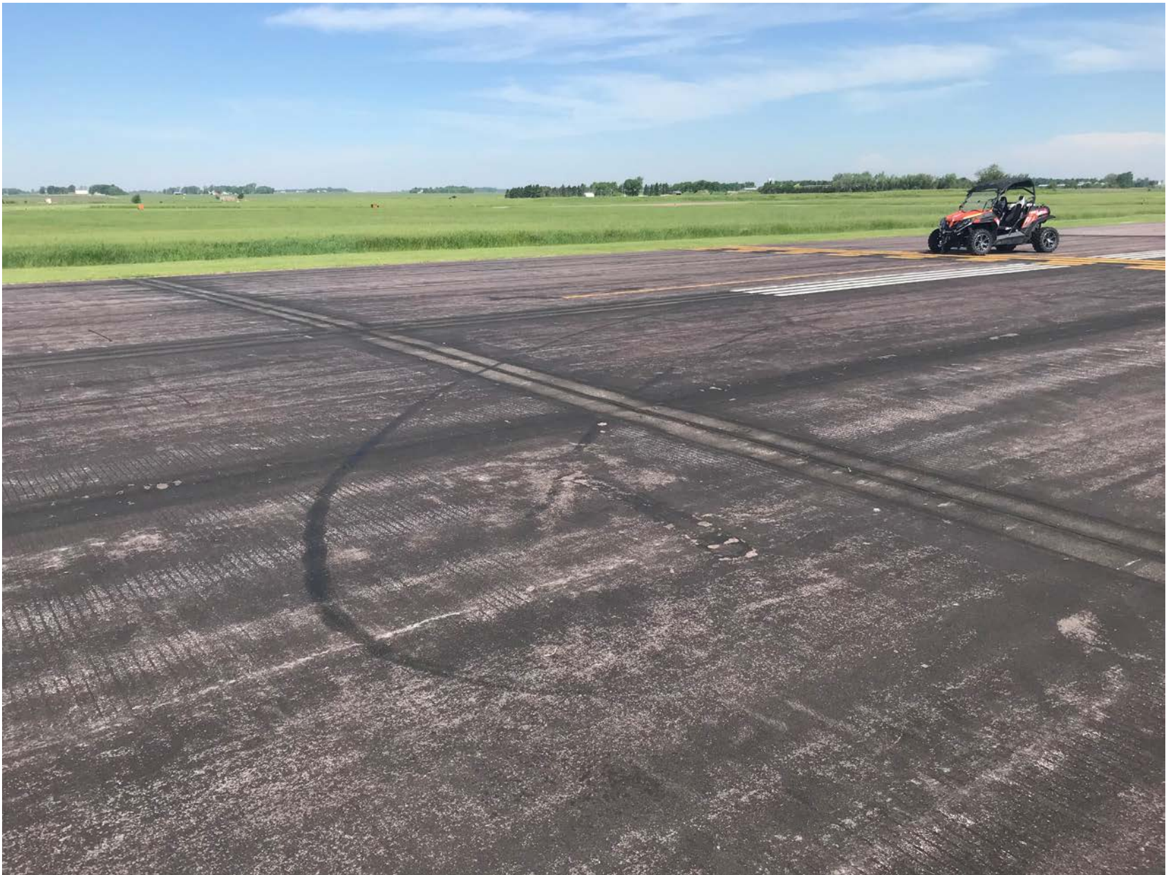
Photo 1 – Tire marks on runway from ground loop
