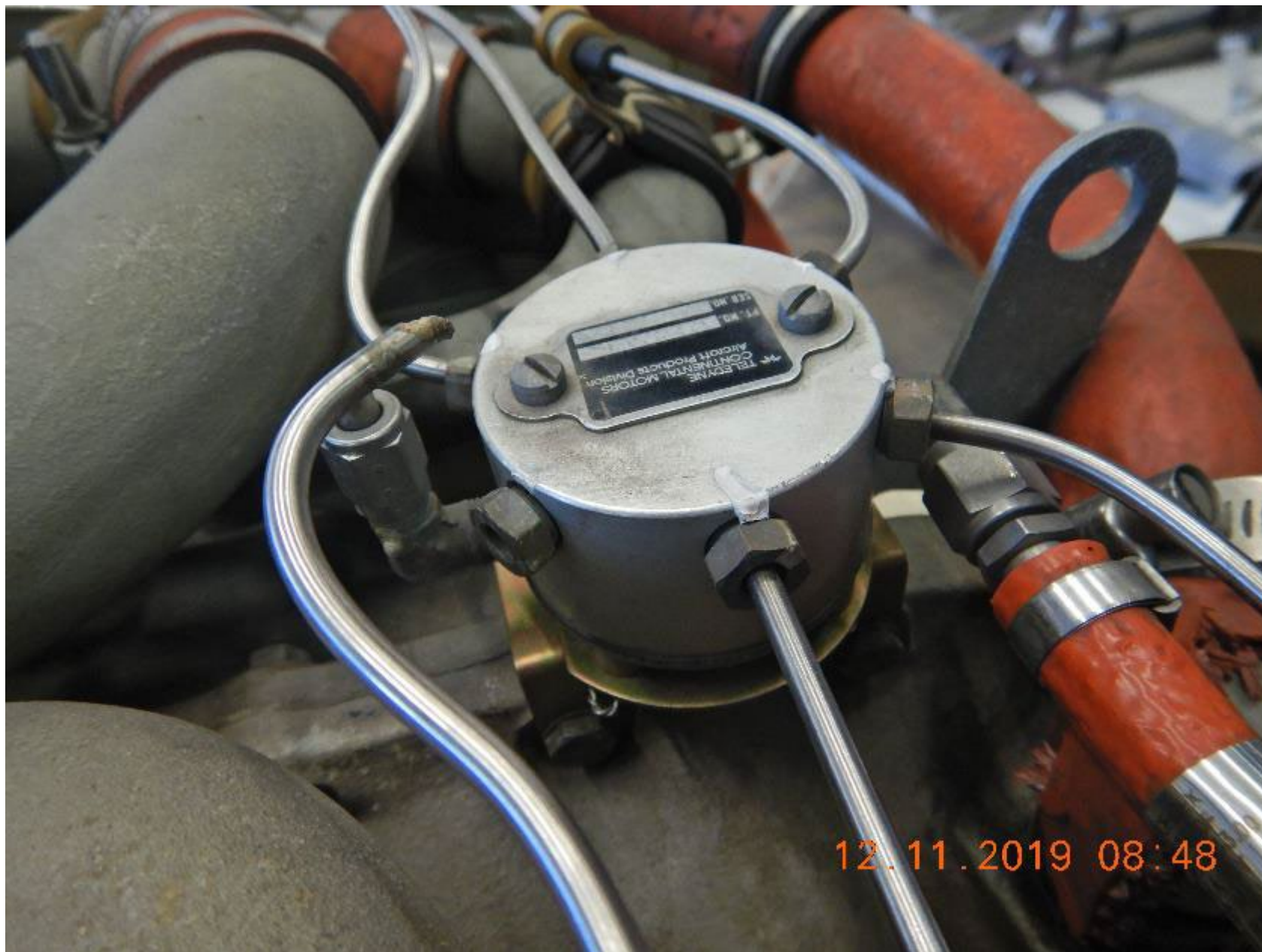
Photo 2 – Broken Fuel Line (Continental Motors Photo)
