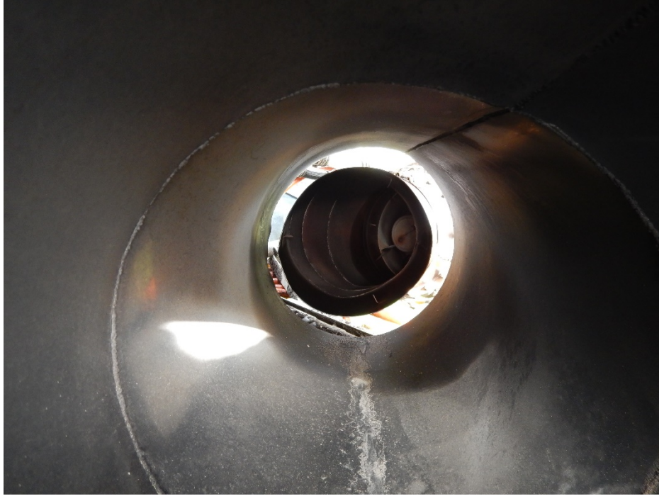
Photo 36 – Eductor Interior Surface – Oil Wetted near Exhaust Duct
