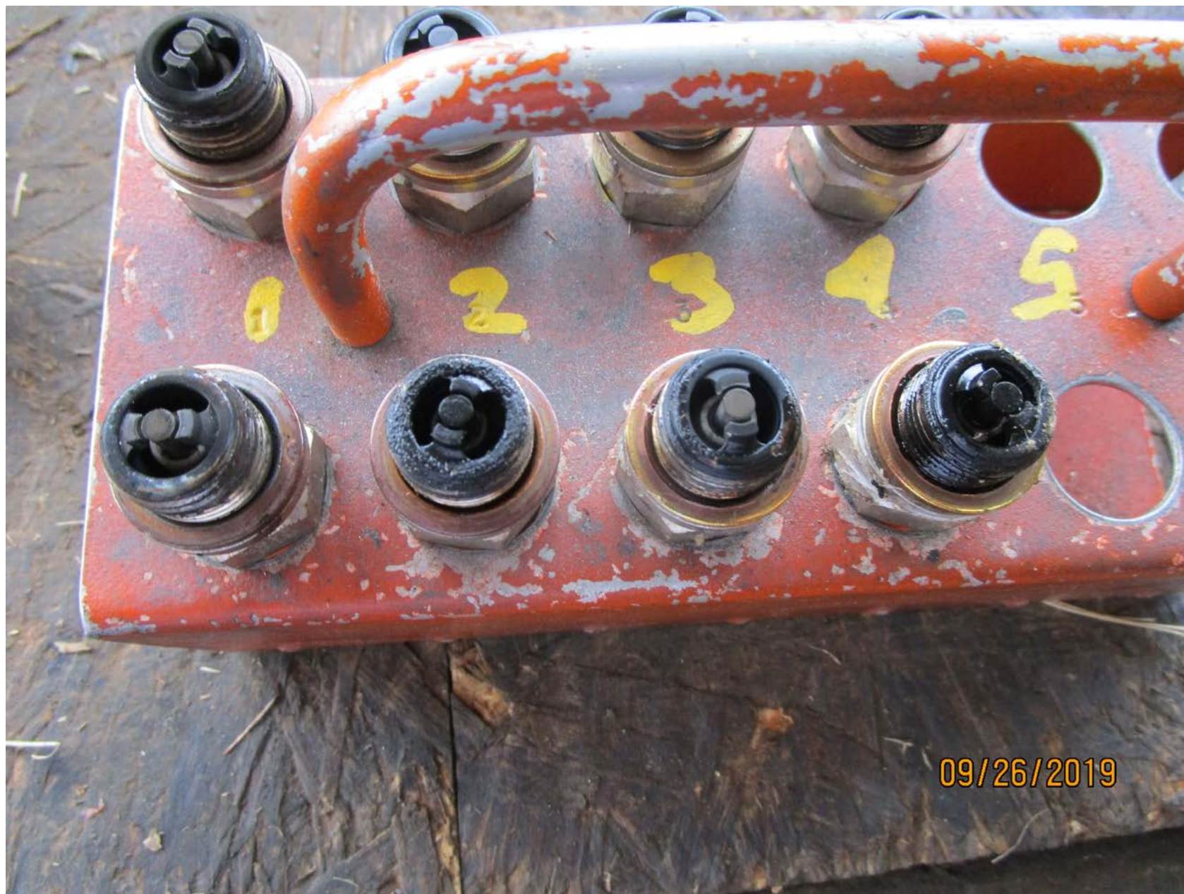
Photo 14 - Close-up view of removed sparkplugs.
