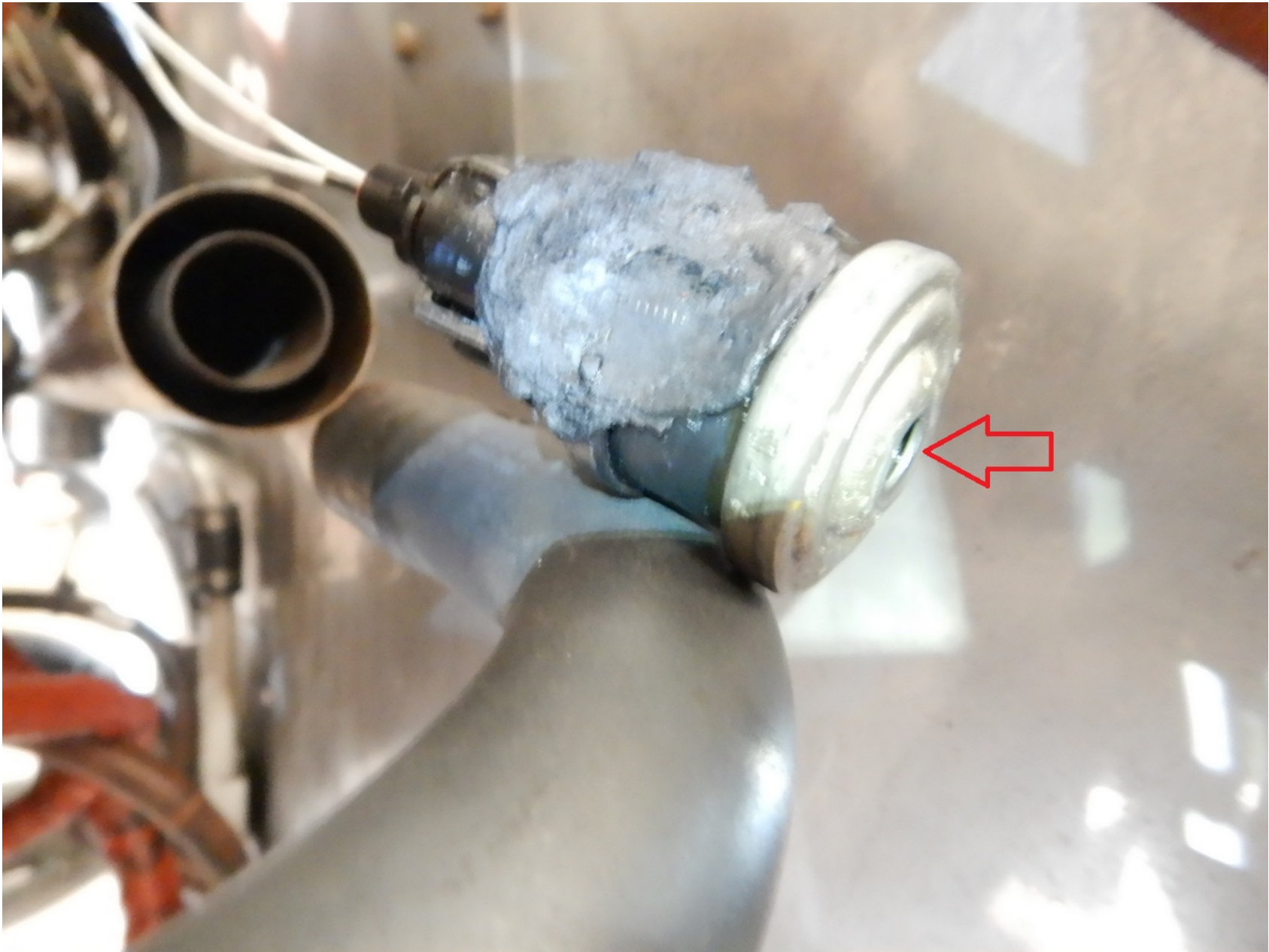
Photo 2 – Oil Pressure Switch with heat damage
