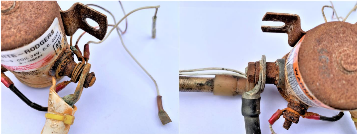
Figure 1. Battery contactor terminal for the positive battery cable was loose (left photo). The battery contactor terminal for the battery switch and starter motor contactor cables was tight (right photo).
