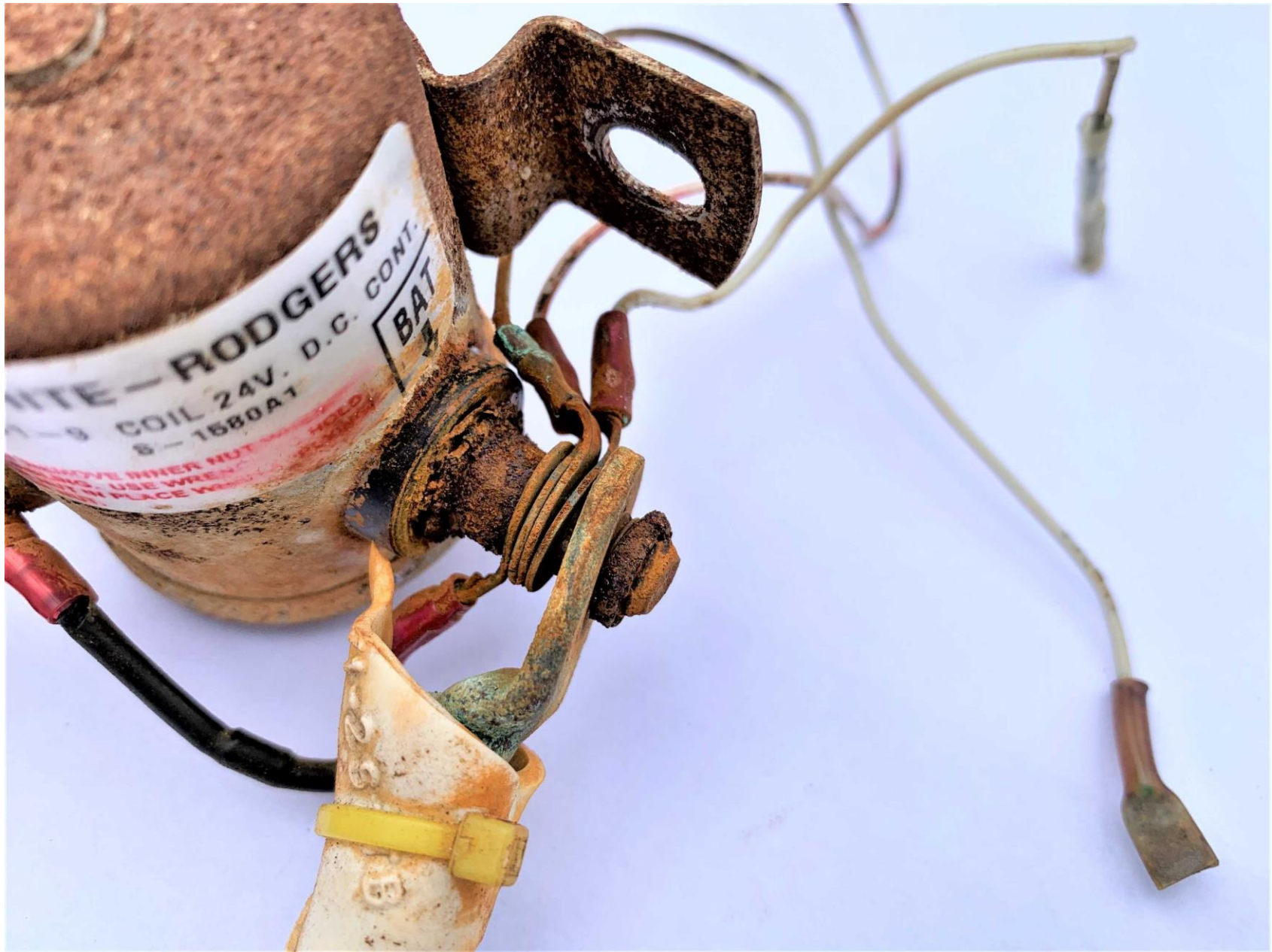
Photo 5 - Battery Contactor Terminal for the Positive Battery Cable
