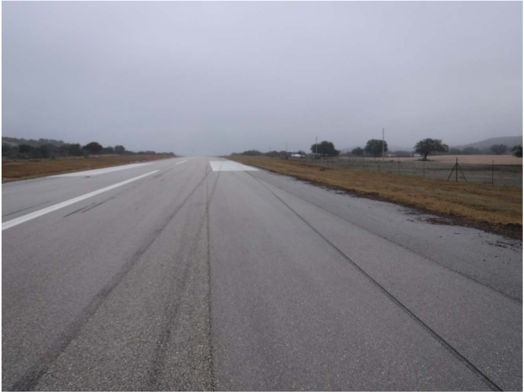
Photo 10 – Runway Excursion Tire Marks, Photo courtesy of Lone Star Retrieval
