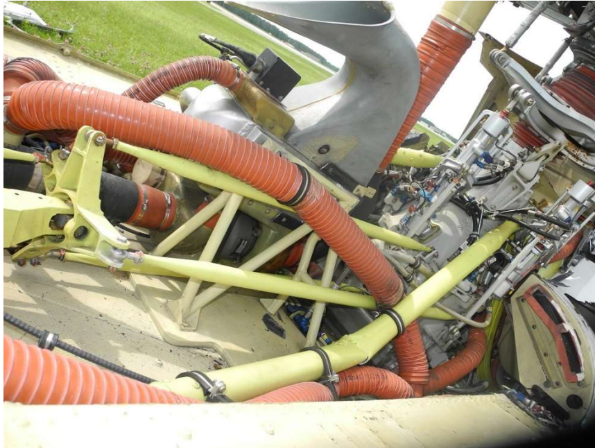
Figure 6. A view of the flight controls from the mixing star to the main rotor hydraulic actuators (only the left and right actuators are visible).
