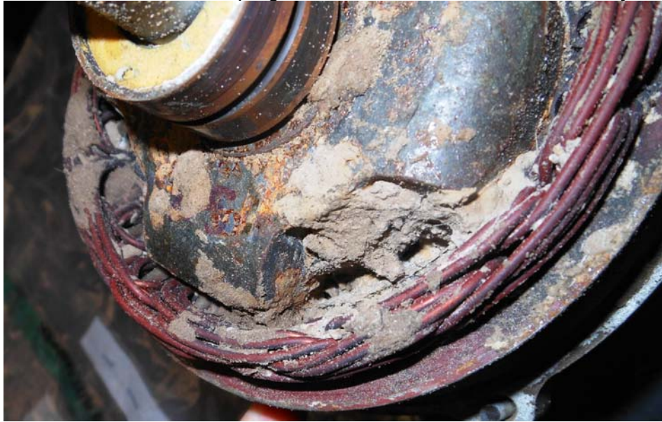
Photo #9 – Rotor impingement on stator/armature assembly
