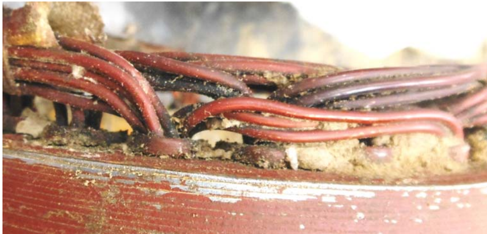
Photo #12 – Some discoloration on stator/armature wires
