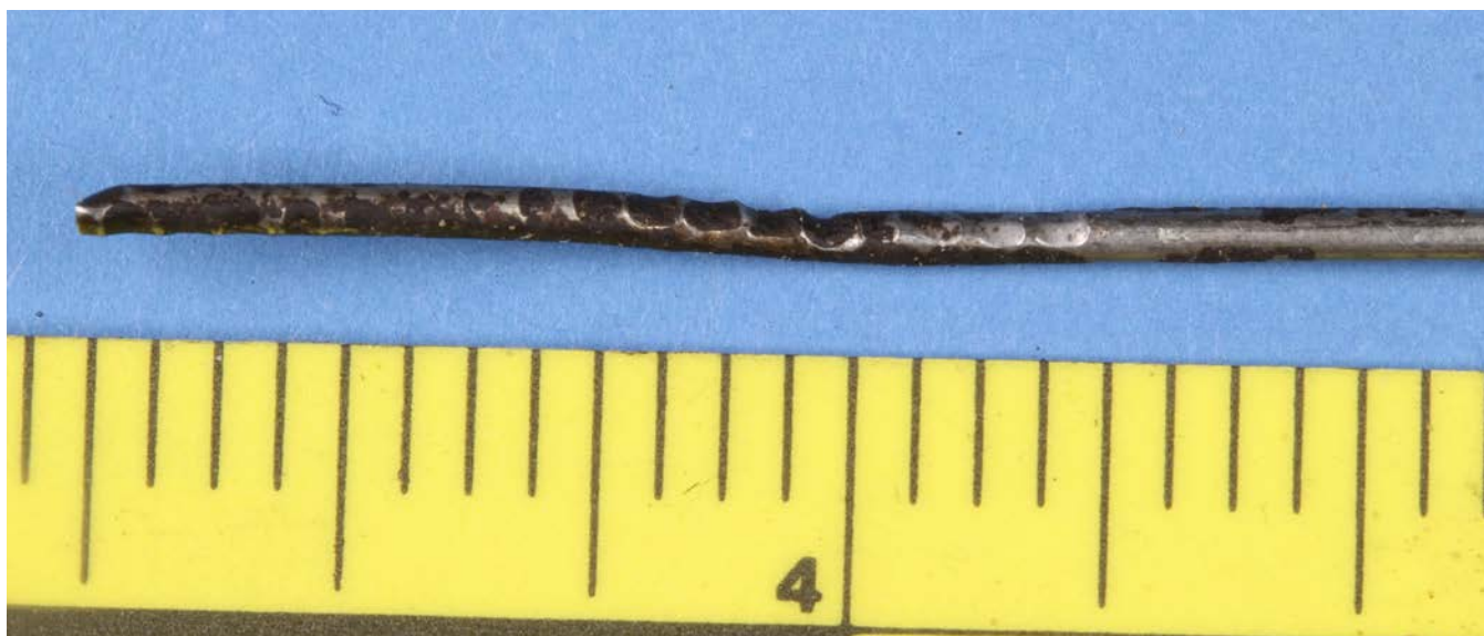
Figure 4: Heat valve shaft control cable end.
