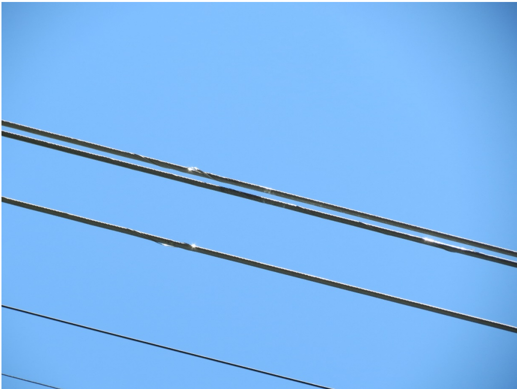
Figure 4: Impact Damage to High-Tension Power Lines
