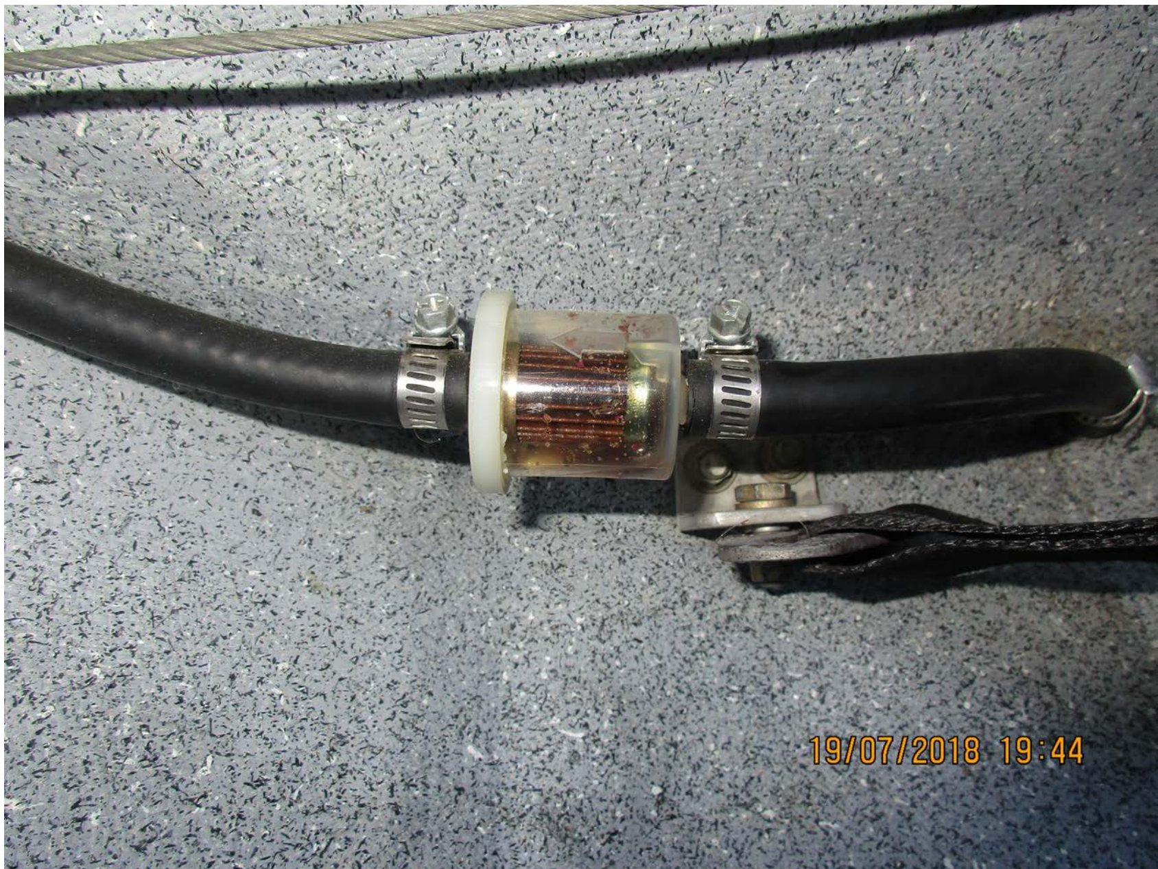
Photo 5 - FAA supplied close up photo of the fuel filter.
