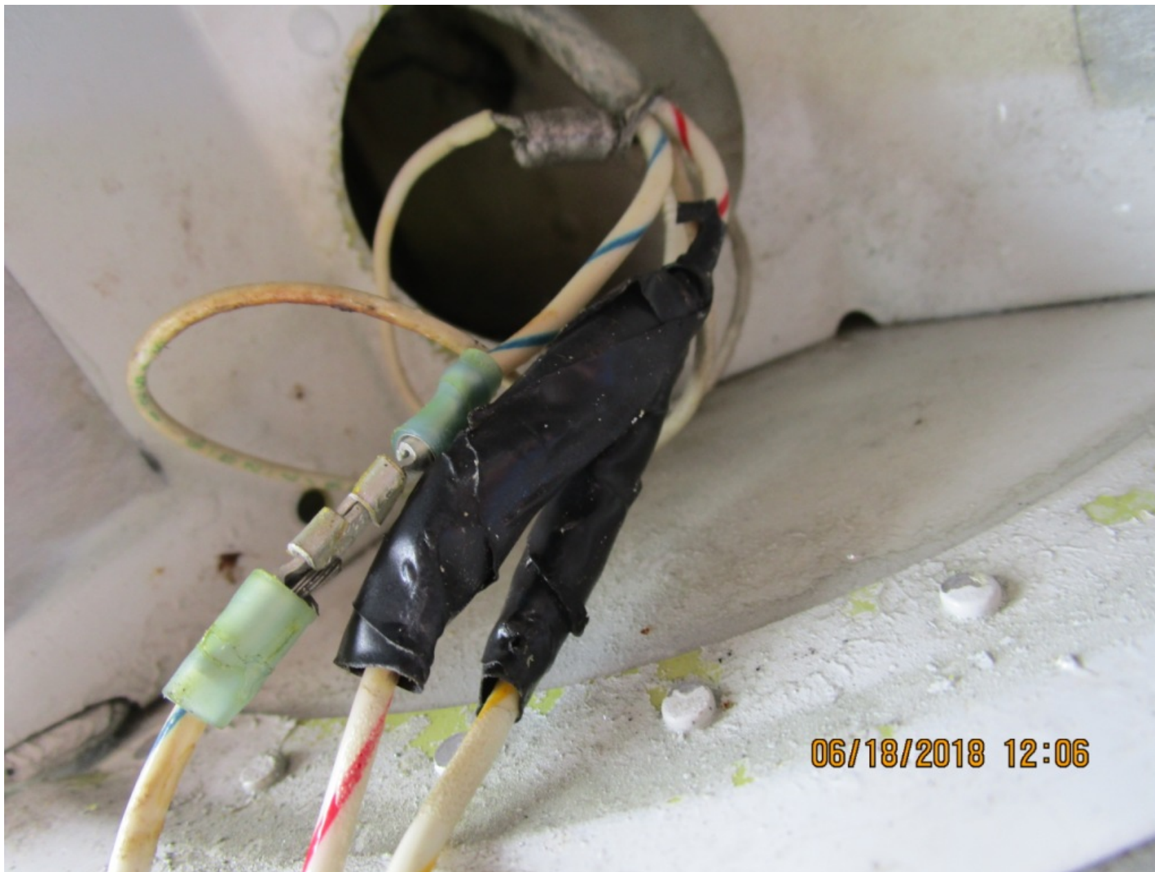
Photo 15 - View of the wiring wrapped in electrical tape (FAA Photo)
