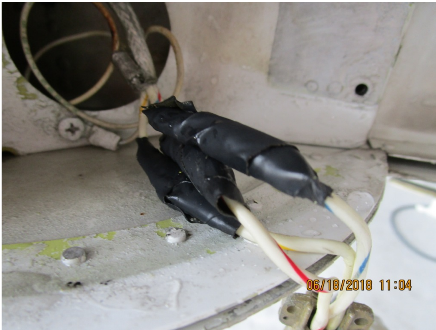
Photo 14 – View of the wiring wrapped in electrical tape (FAA Photo)
