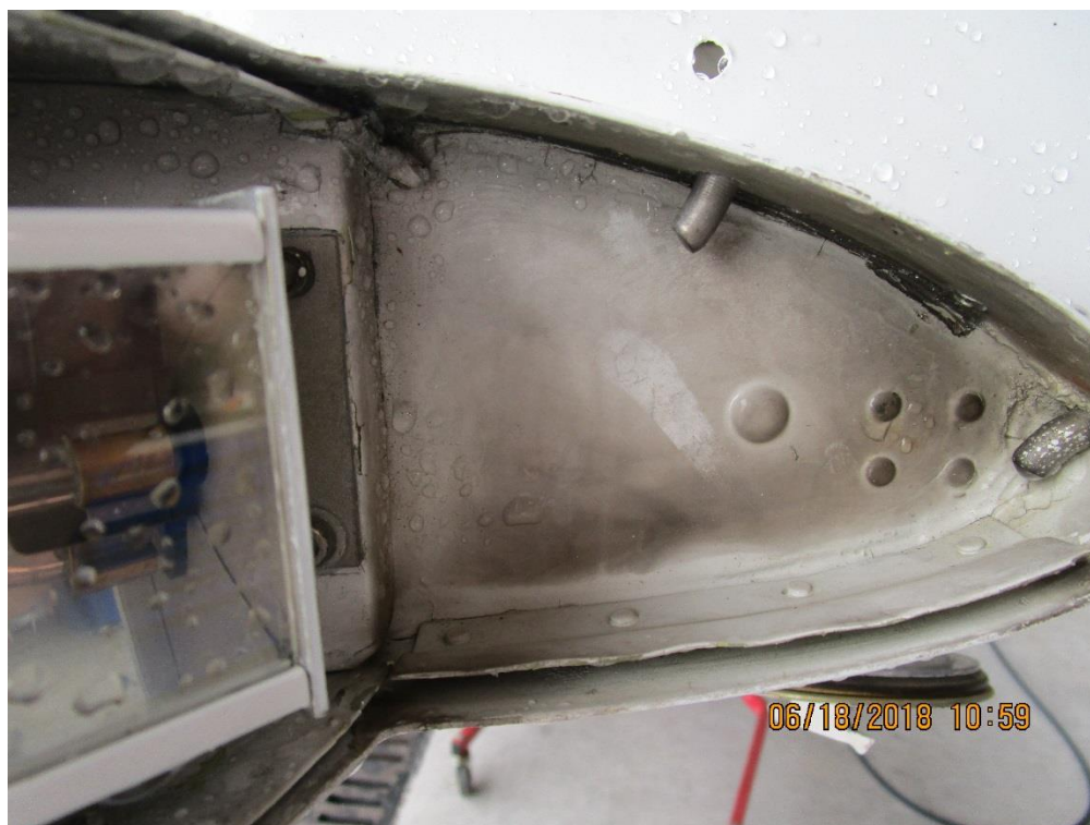
Figure 5 1603 Soot on bulkhead.
