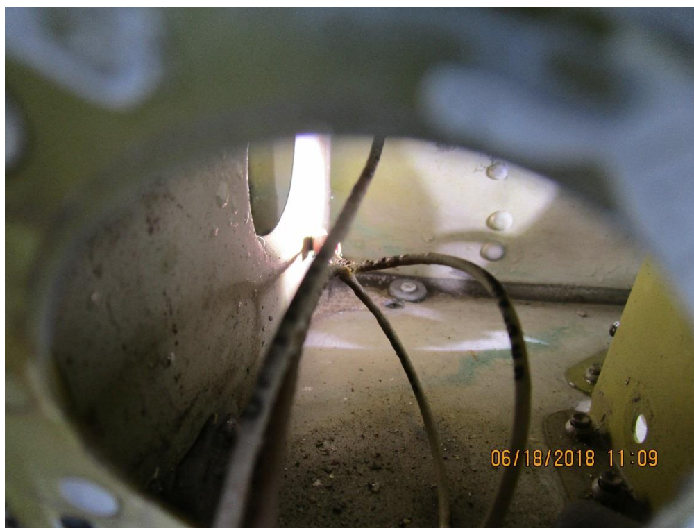
Figure 4 1608 Navigation light wiring slightly burned.
