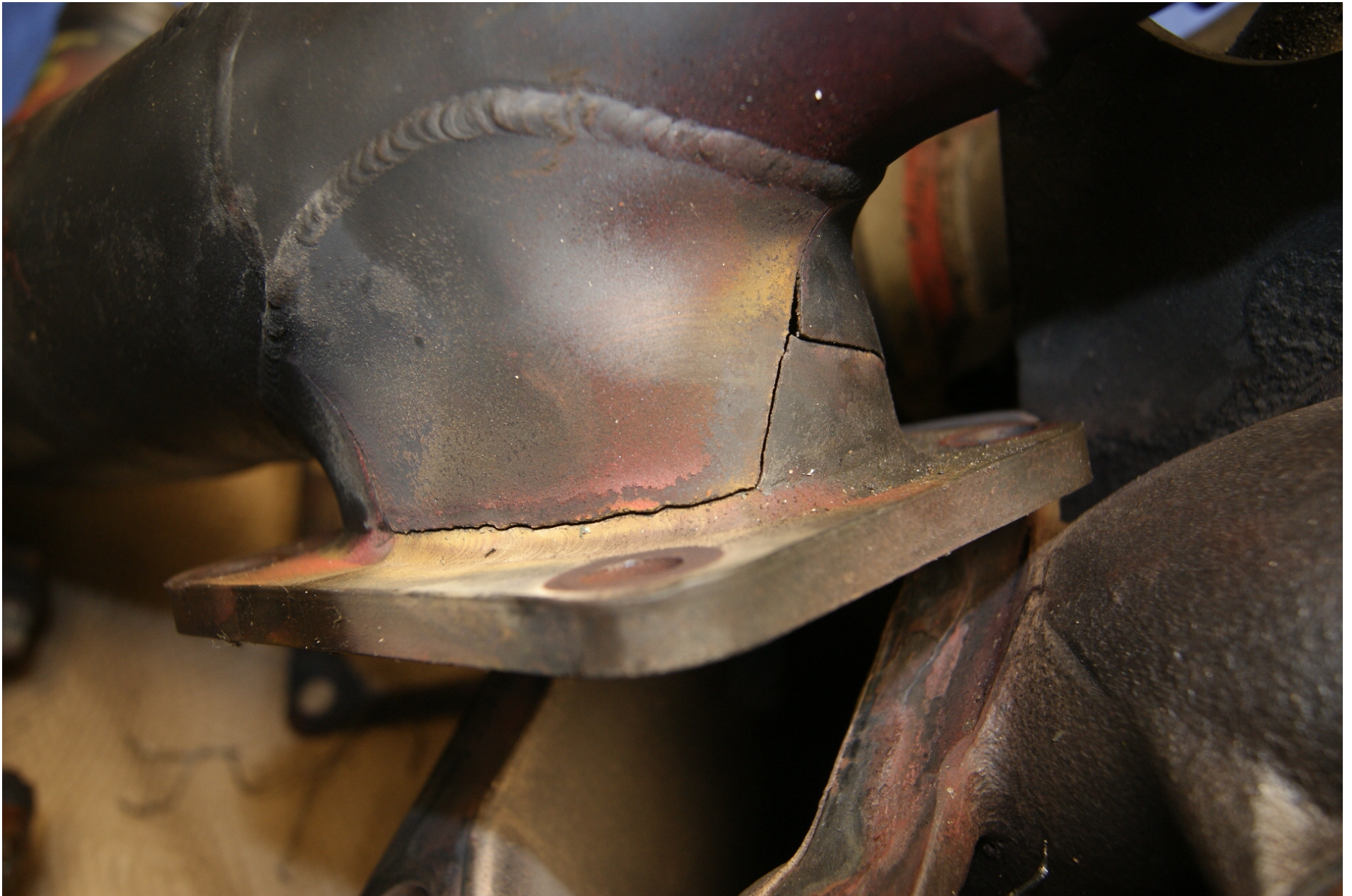
Photo 3 – Crack at the base of the manifold.
