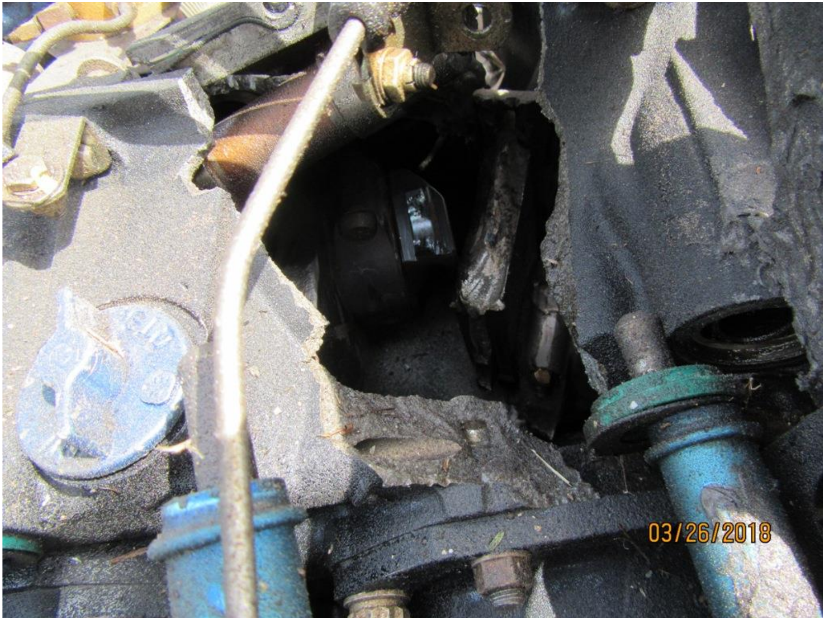
Photo 3 – Hole in Engine on N540JH
