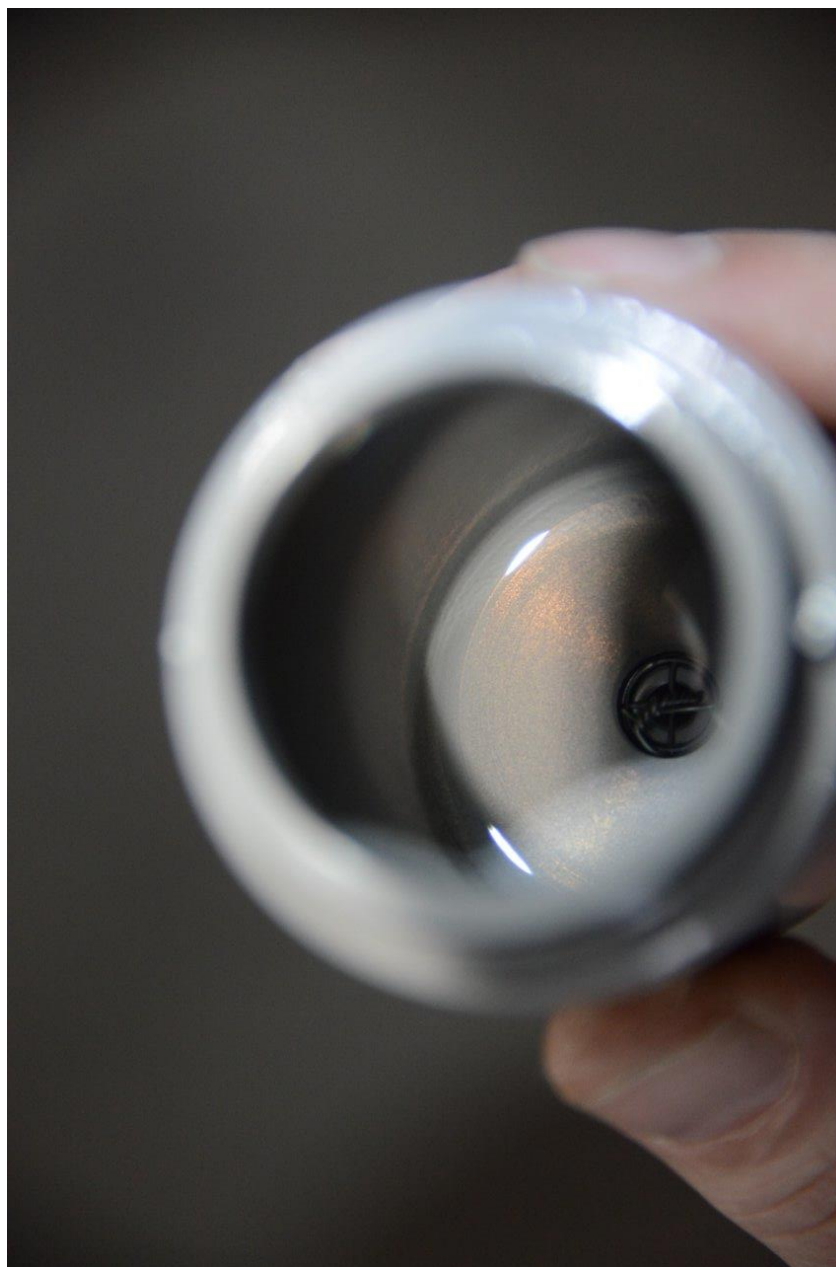
Photo 7 - View of the fuel filter bowl with a liquid present.
