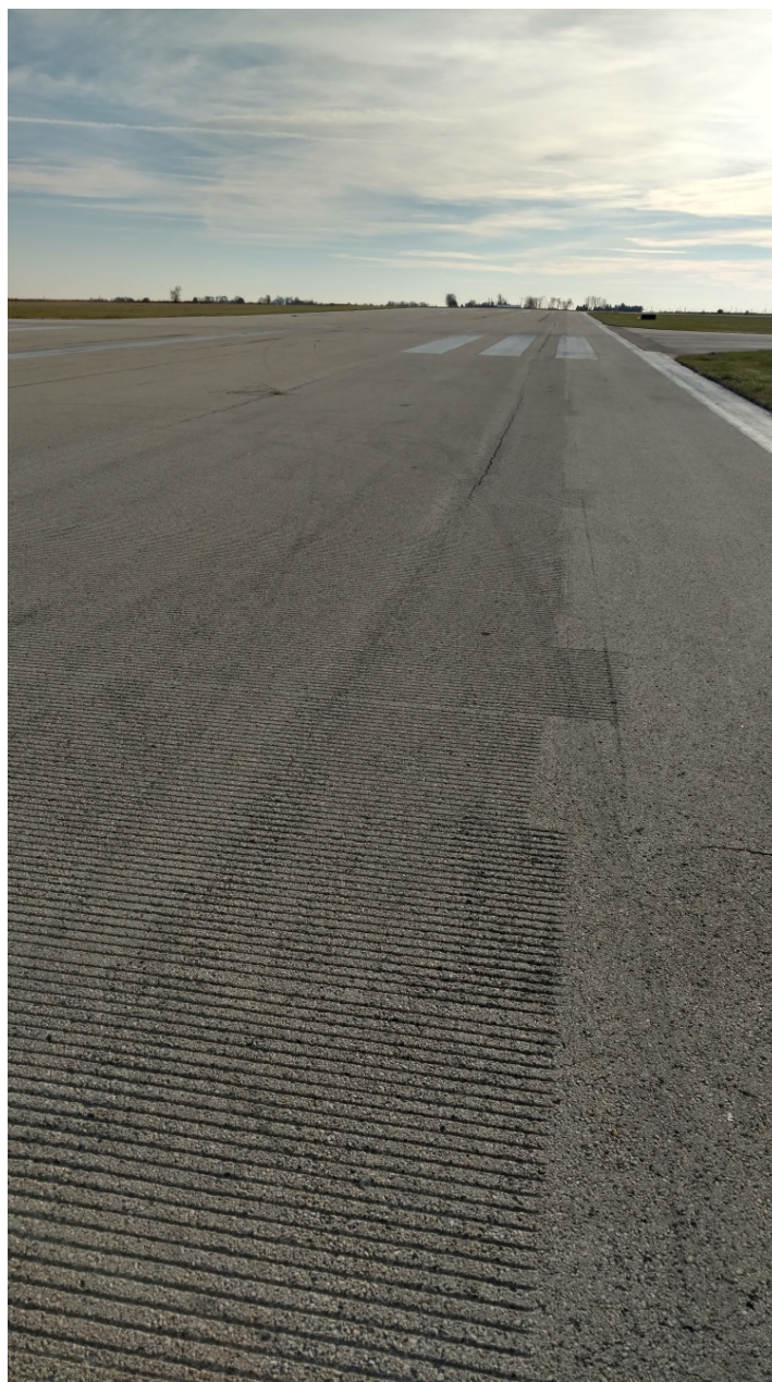
Photo 1 – Tire marks on runway
