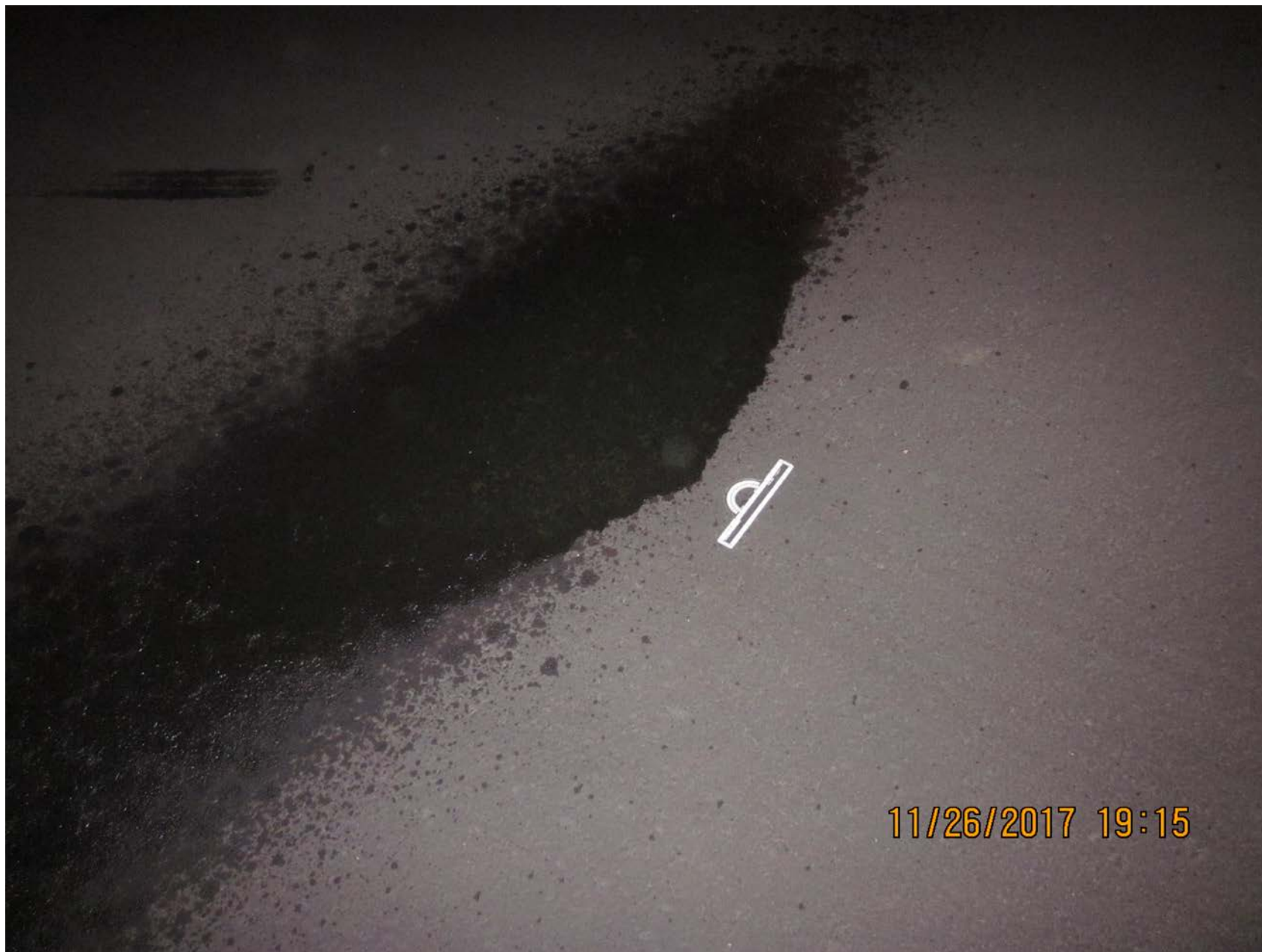
Photo 2 – Oil residue on taxiway
