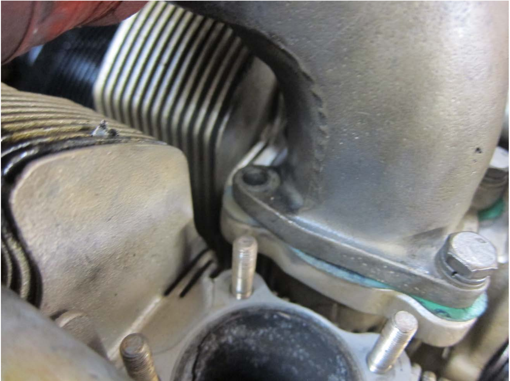
Photo 10 – View of one of the missing induction riser bolts (CM Photo)
