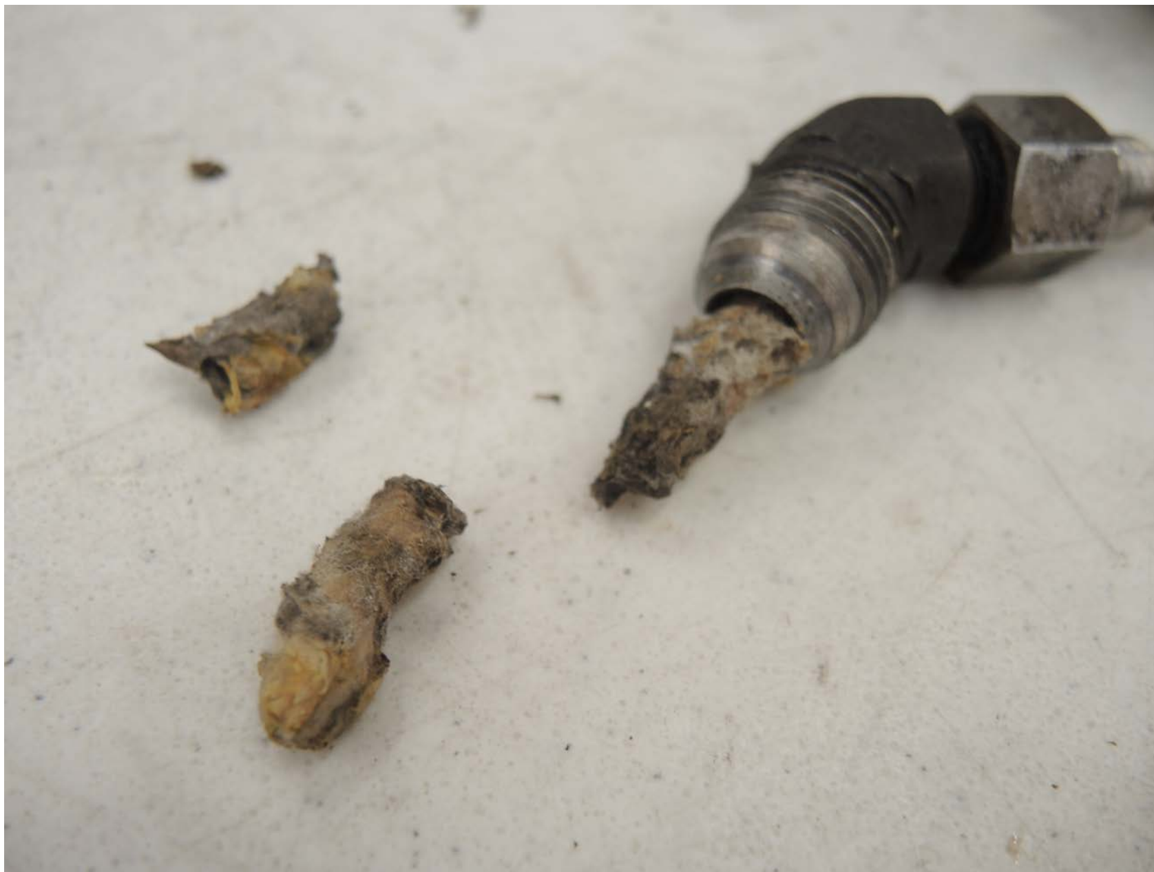
Photo 17 - Organic Debris In Fuel Fitting
