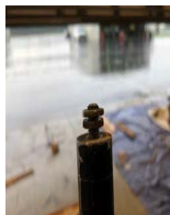
Image 6: Side View – Severed Rod End
