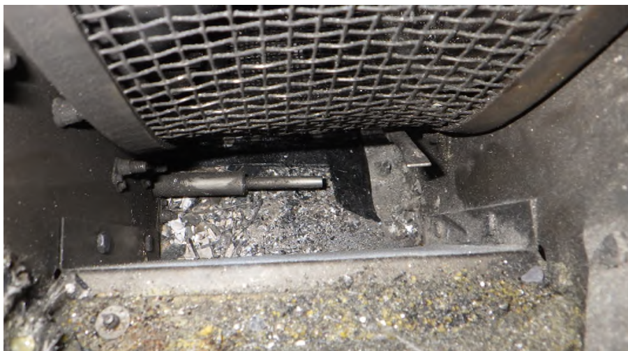
Photo No. 53: Debris and soot in the inlet
