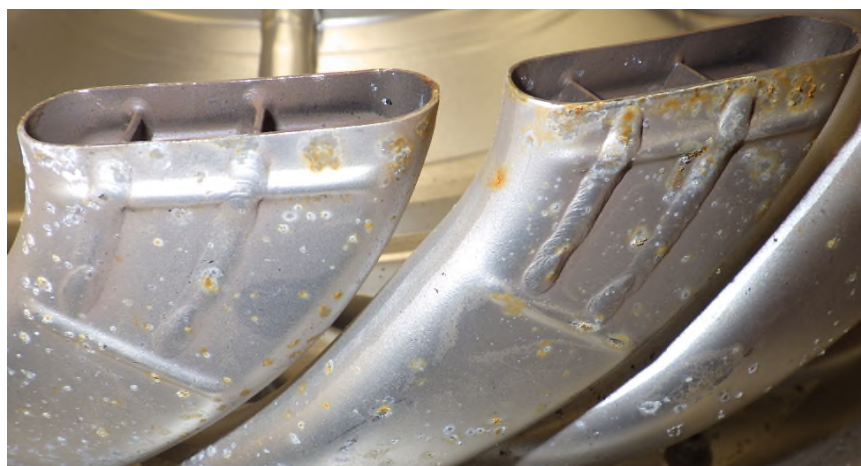
Photo No. 13: Diffuser pipes
