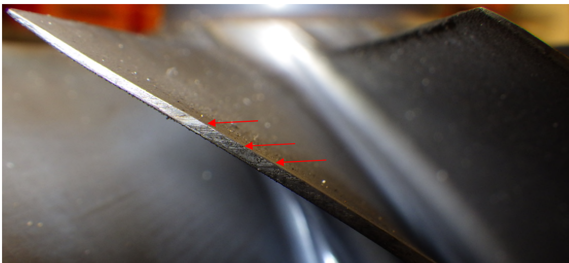
Photo No. 9: Centrifugal impeller rubbing
