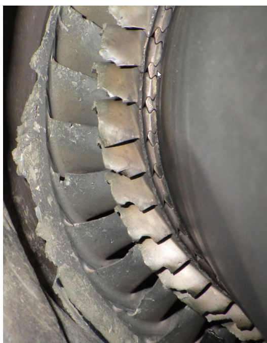
Photo No. 80: PT blades fractured
