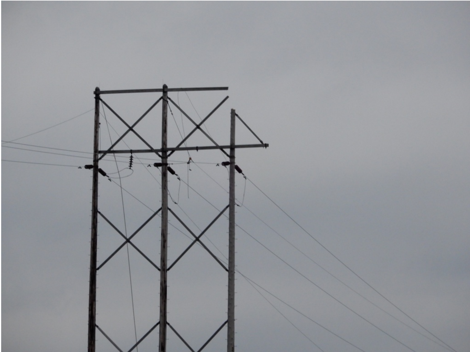
Photo 12 – Broken Pole Structure and Lines
