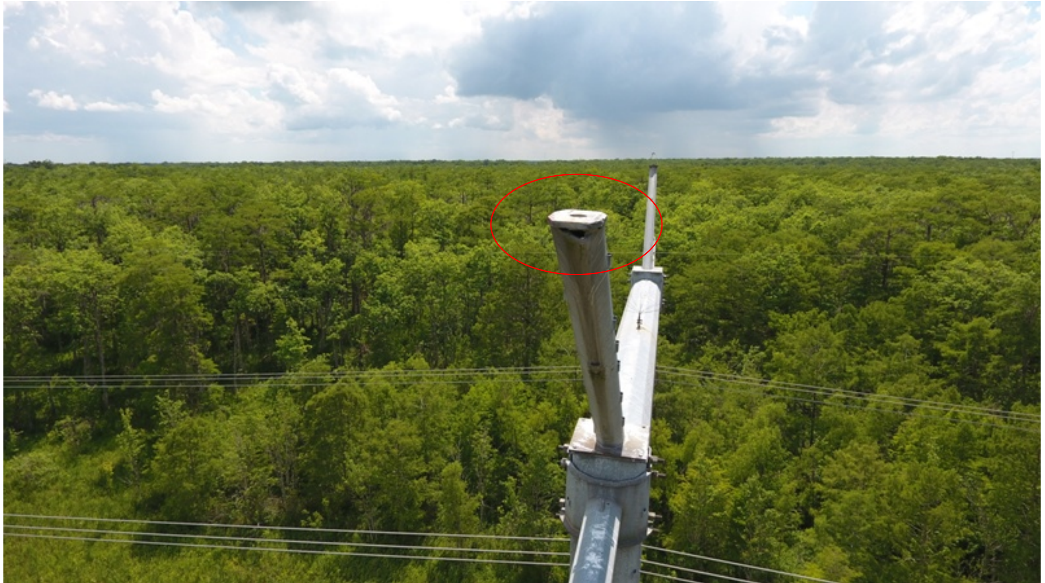
Structure arm after the accident showing a missing bracket and damage under top plate.
