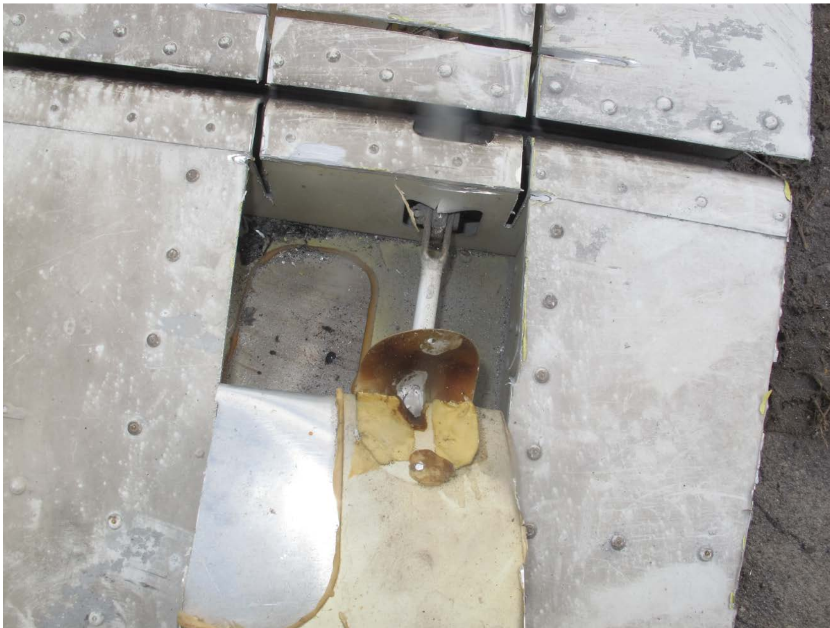
Photo 12 – Elevator Trim Control Rod
