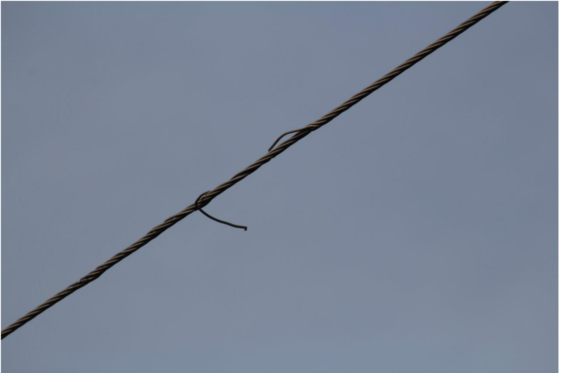
Photo 20 - Close-up view of a powerline with a separated strand.
