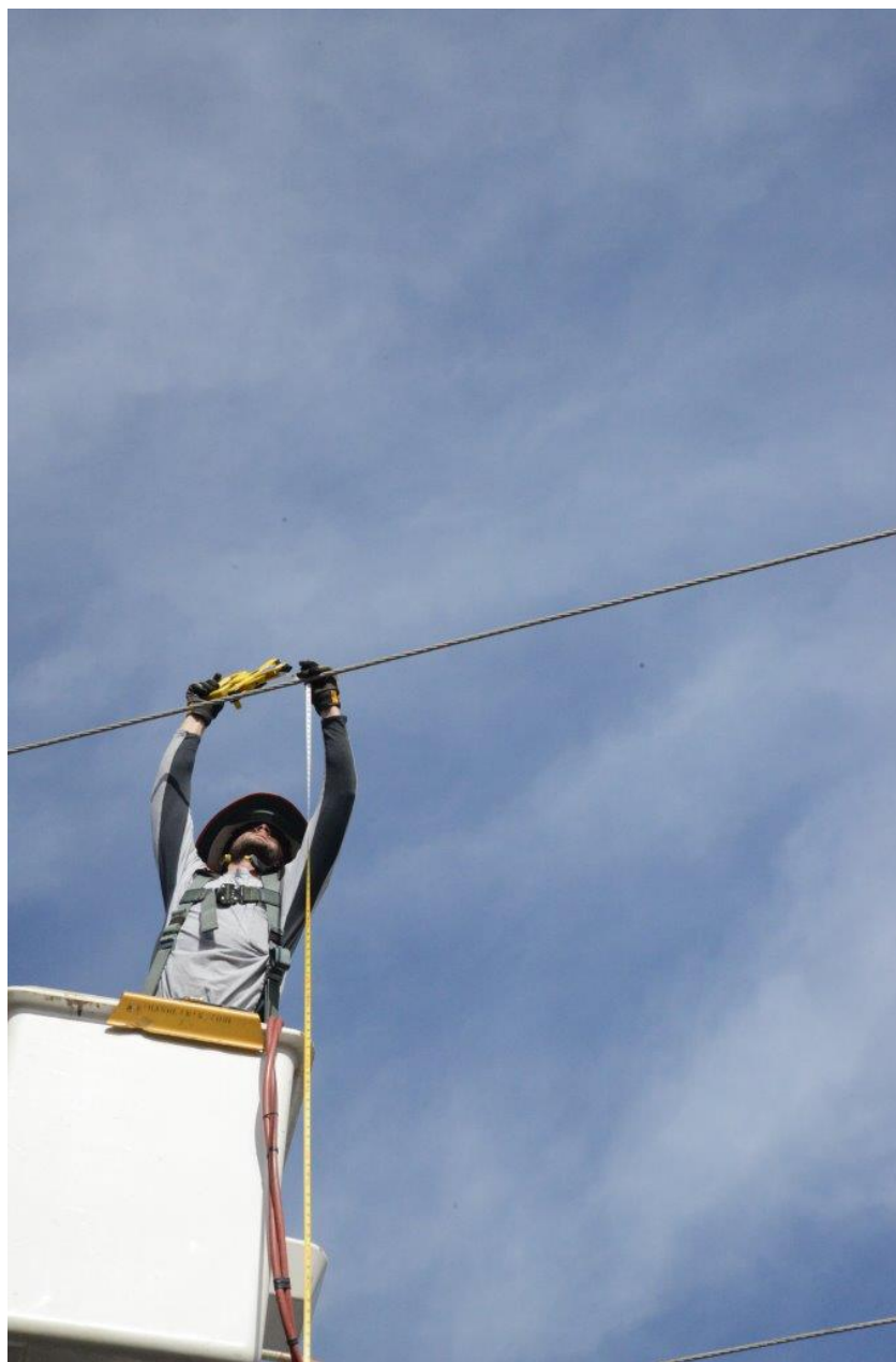
Photo 18 - Powerline personnel measuring the height of the powerline at the accident site.
