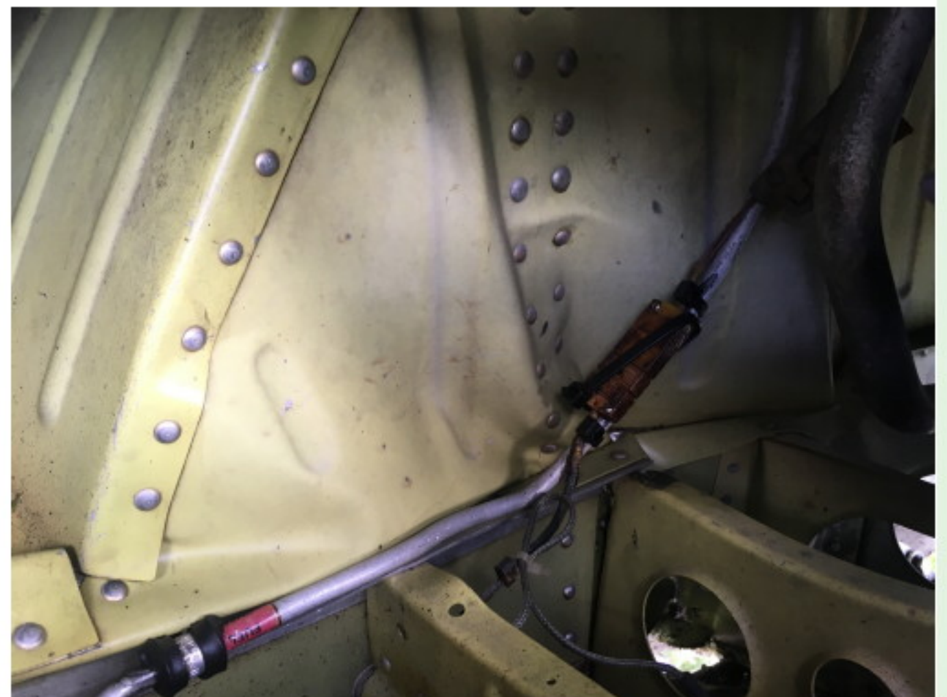
All support structure will require replacement
