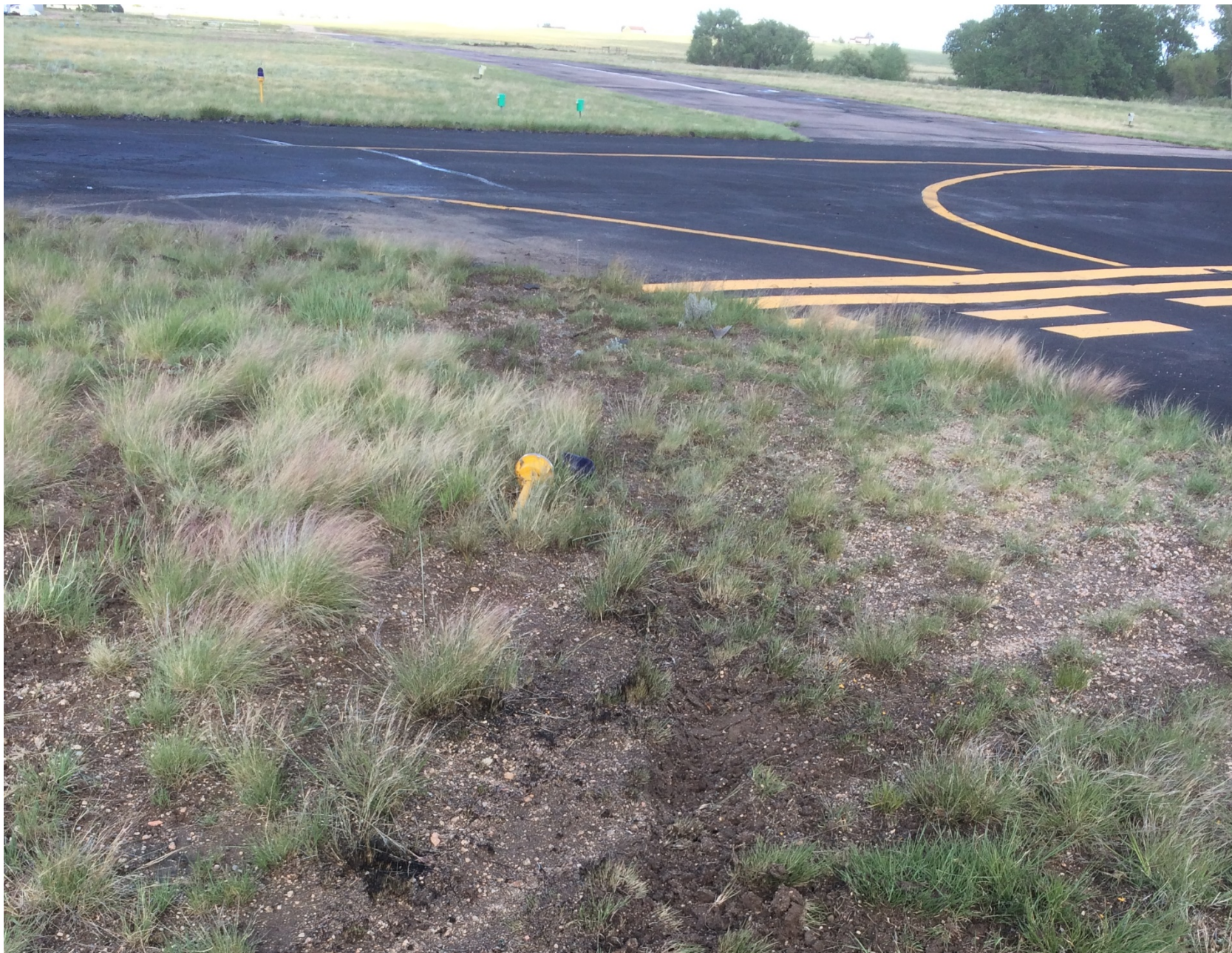
Photo 2 –Area Preceding Taxiway Light
