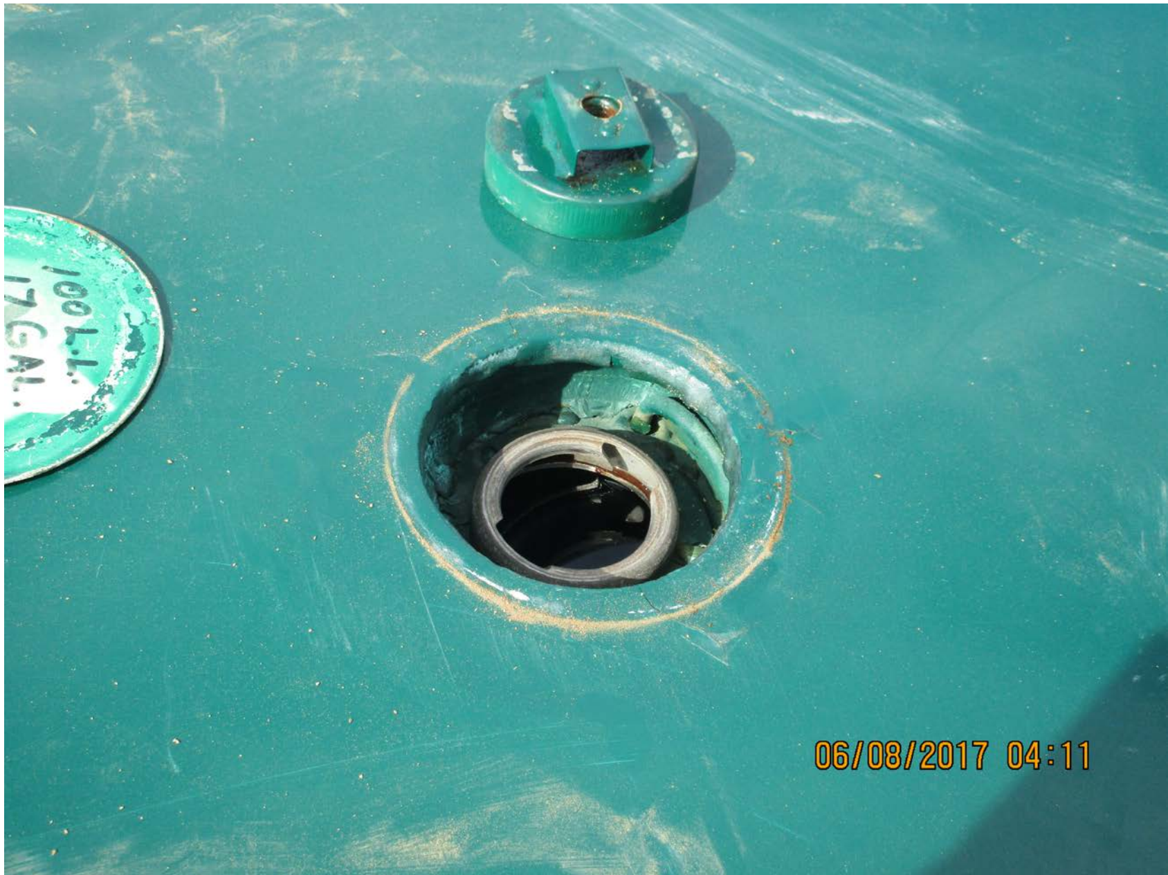
Photo 5 – Right auxiliary tank port
