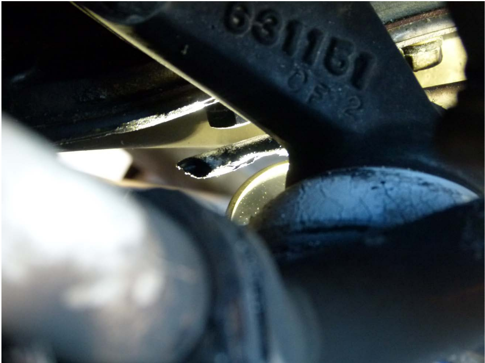
Photo 2 - View of burnt drain line
