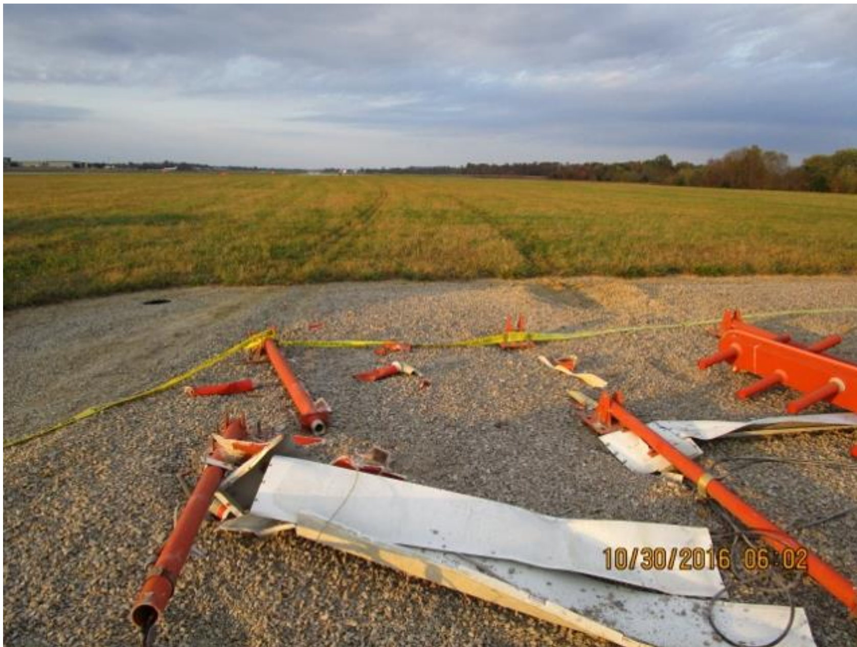
Photo 5 – View of the damaged ILS structure looking back at the runway
