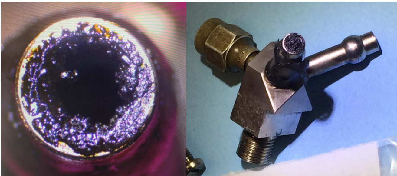
Figure 20/21 – No. 2 deck fitting opening for vent tube clogged with coke
