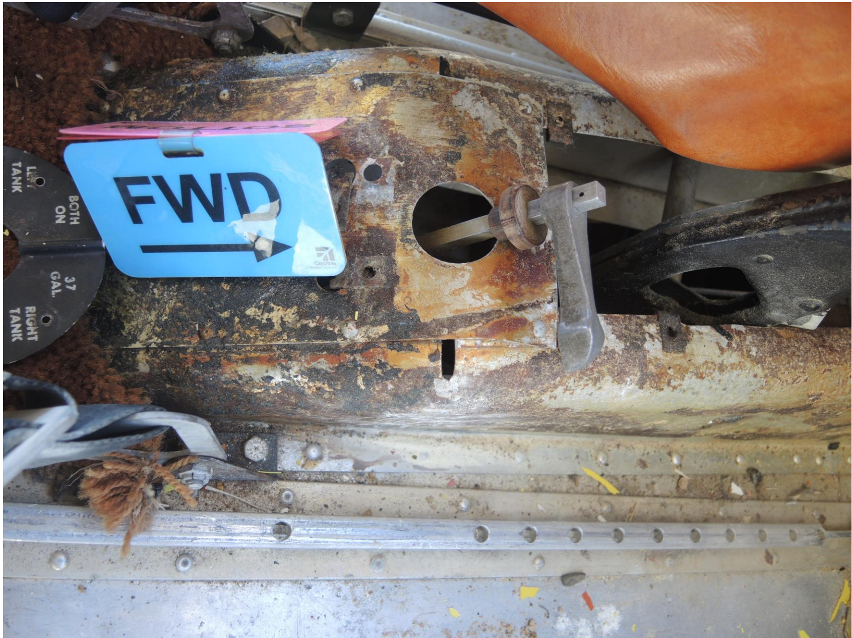
Photo 1 – Textron Aviation supplied image of the fuel selector. The selector lever is pointed to the right tank position.
