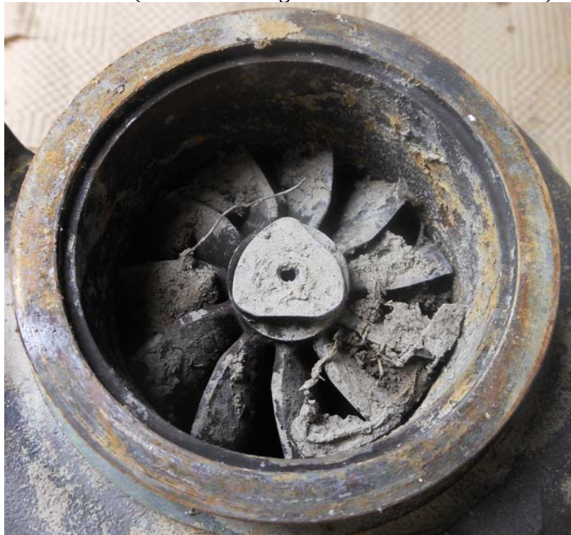
Photo #17 (Left Turbocharger Turbine Wheel and outlet)
