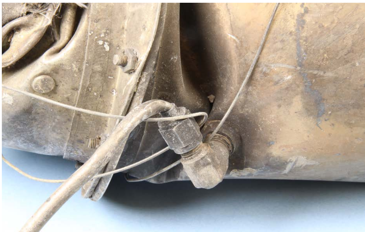
Figure 6: Loose fuel fitting near ventilation air inlet side of combustion heater body.
