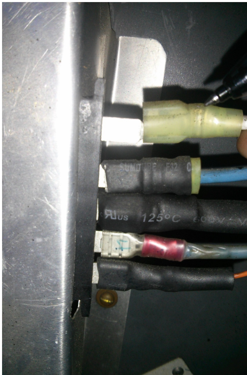
Photo 1 – View of the Voltage Regulator supplied by the Pilot.
