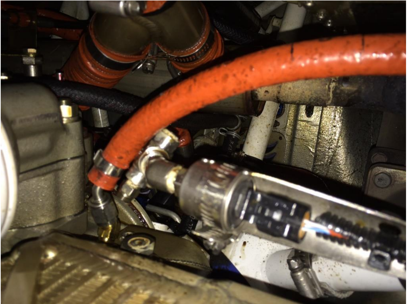
Photo 5 – Broken Cross Fitting
